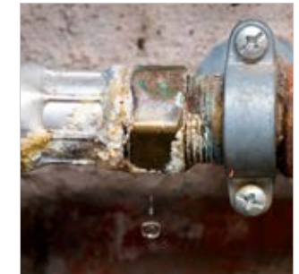
BOILER LEAKS CAN WASTE ENERGY AND ARE EASY TO FIX
